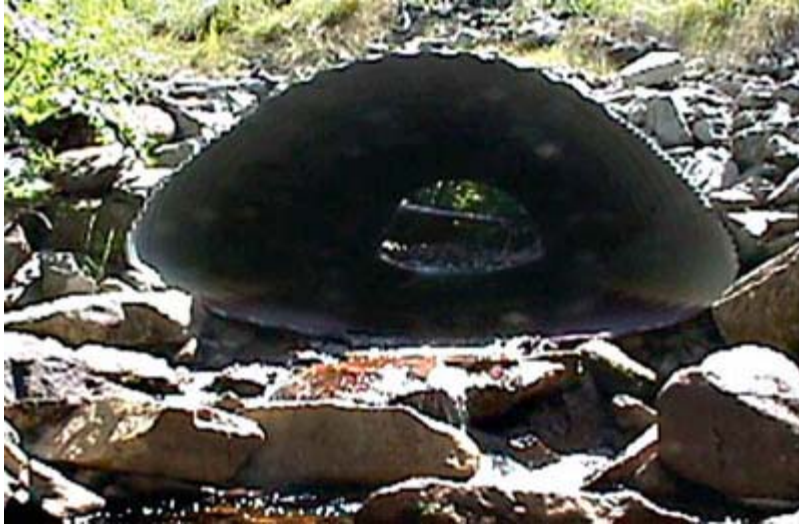
Figure 6.6 Downstream riprap will dissipate energy and reduce scour, but must be placed with fish utilization in mind (USFS 2005)
