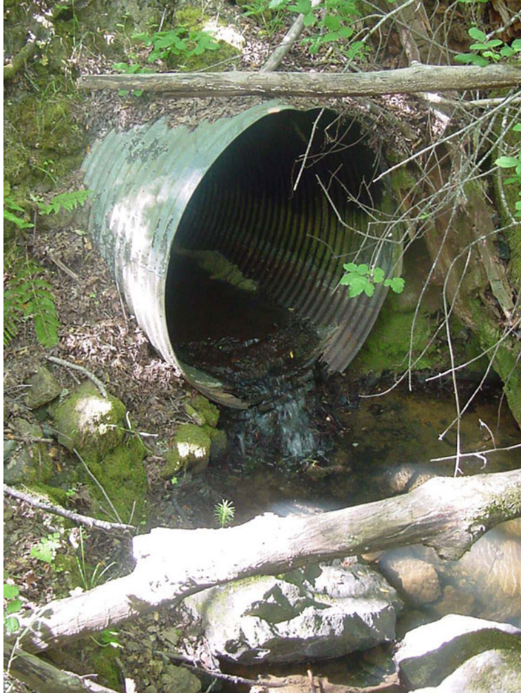
Figure 8.13 Pre-existing outlet of John Hatt Creek culvert perched at 0.46 m (1.5 ft) blocks migrating steelhead
