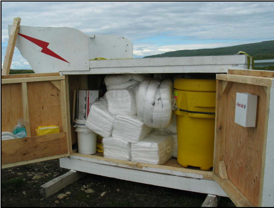
Photo #54. White container full of spill equipment. A first aid kit is on the door to the right.
