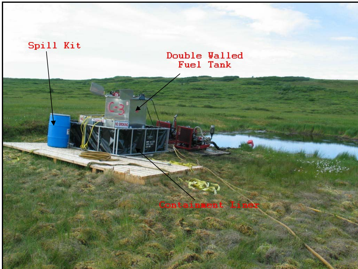
Photo #55. Water pumping facility taking water from a small pond.
