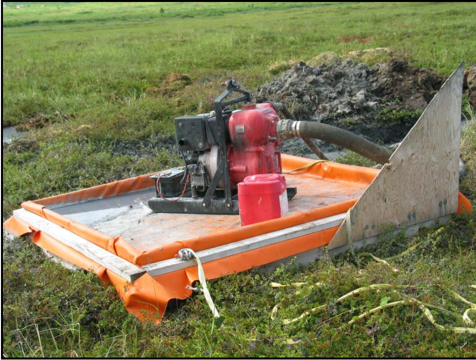
Photo #23. Sump pump at drill #7. Pump is in a containment structure due to proximity to wetland.
