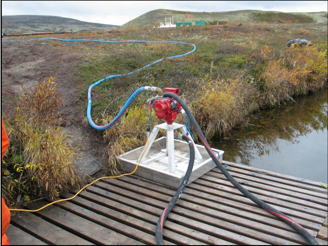
Photo #15. Electric pump on dock at Big Wiggley fuel storage.
