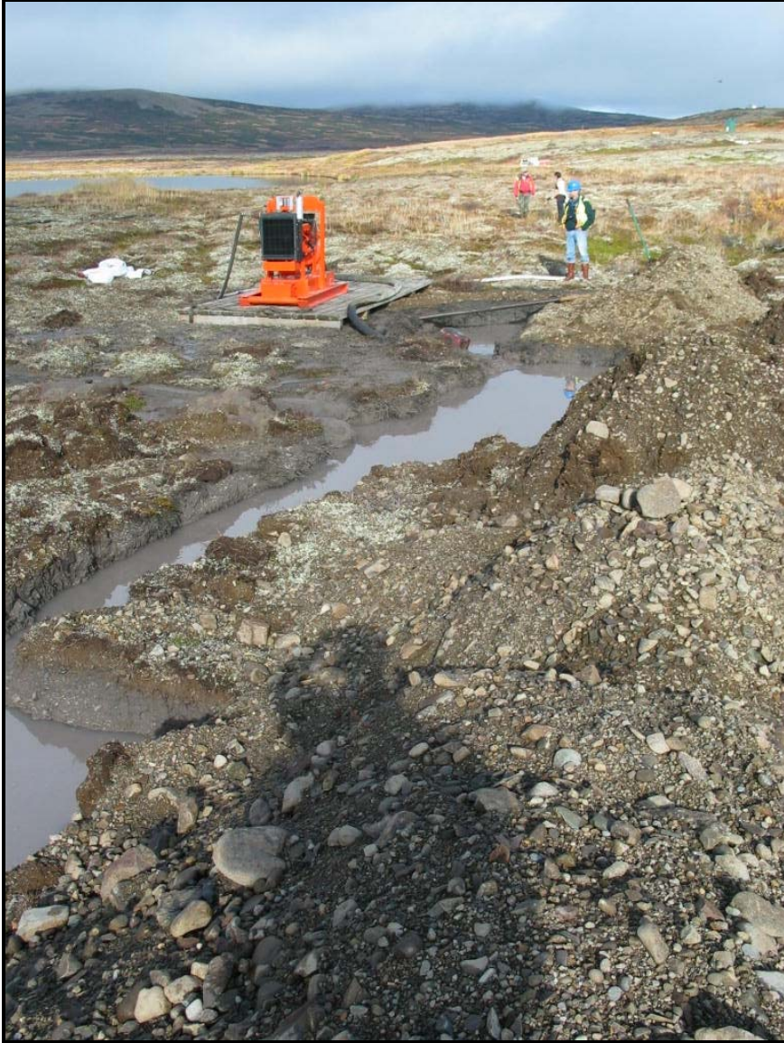
Photo #12. Larger sump required for recirculating fluids at drill #5.
