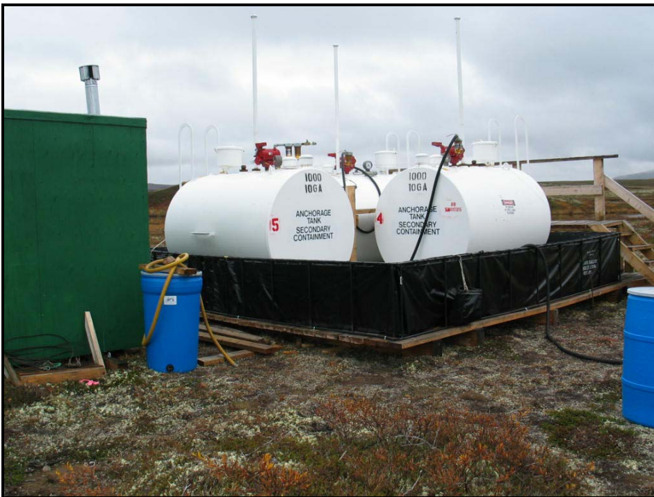
Photo #14. Larger, 3,000 gallon fuel containment at Big Wiggley. Each containment has a large fire extinguisher, spill kit, and scrubber barrel. The facility also has a large container of spill materials.
