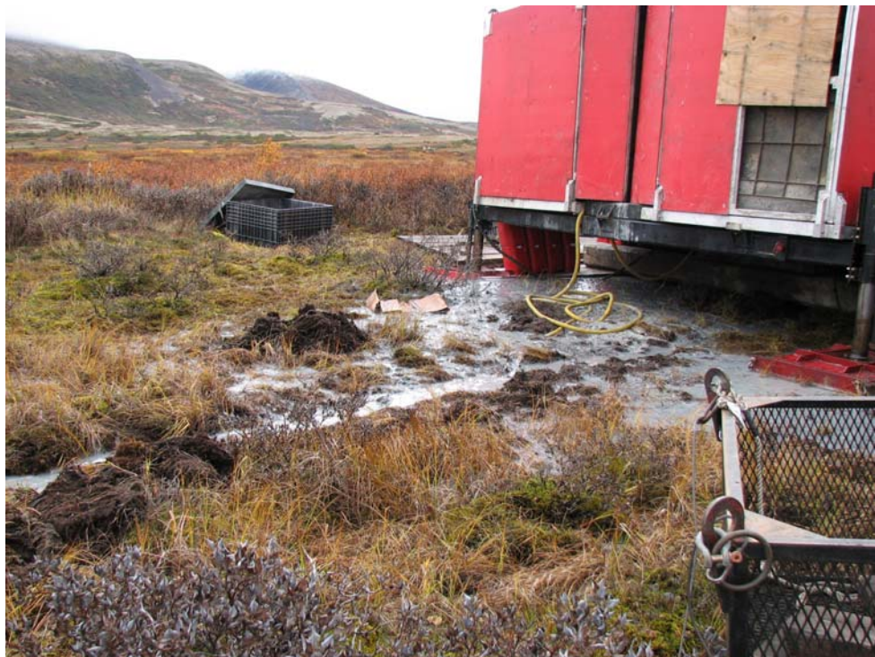
Photograph No. 8: Drill Site No. 7385 Trench and sump pit system is inadequate owing to marshy conditions.
