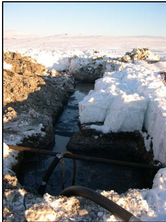
Figure 8. Water recycle sump, drill rig number 5.
