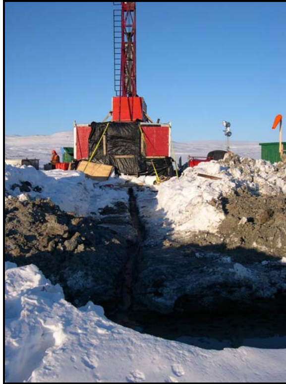
Figure 7. Water recycle sump, drill rig number 5.
