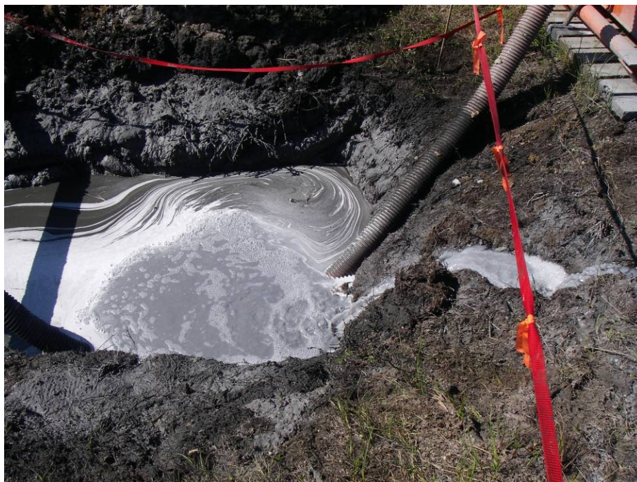
Figure 6. Drill water overflow and recycle sump, drill rig 8412 (No. 6)
