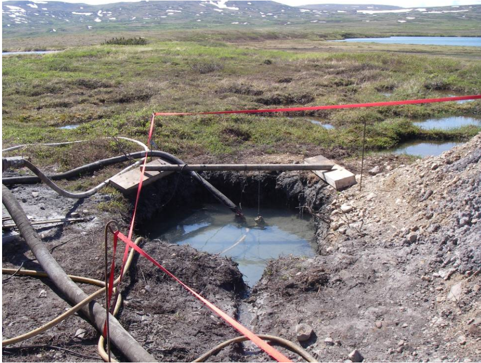
Figure 5. Drill water overflow and recycle sump, drill rig 8407 (No. 5).
