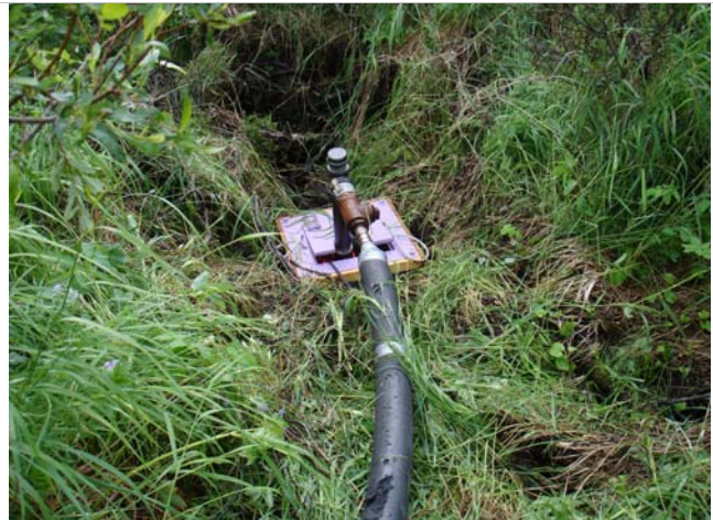
Figure 4. Water intake for drill rig 2.
