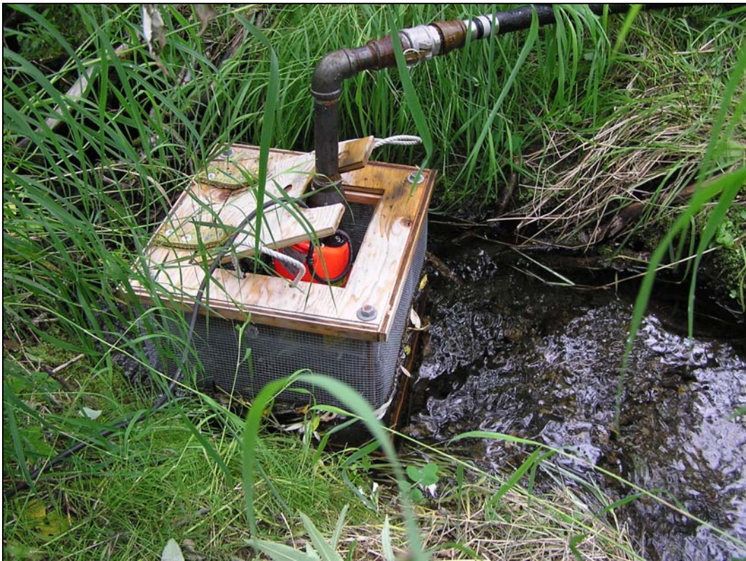
Figure 14: Screened intake for Drill Rig # 2.
