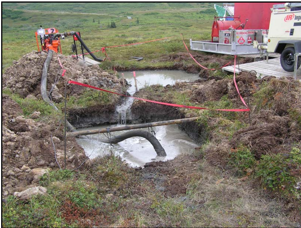
Figure 6: Primary and secondary sumps at Drill Rig # 3.
