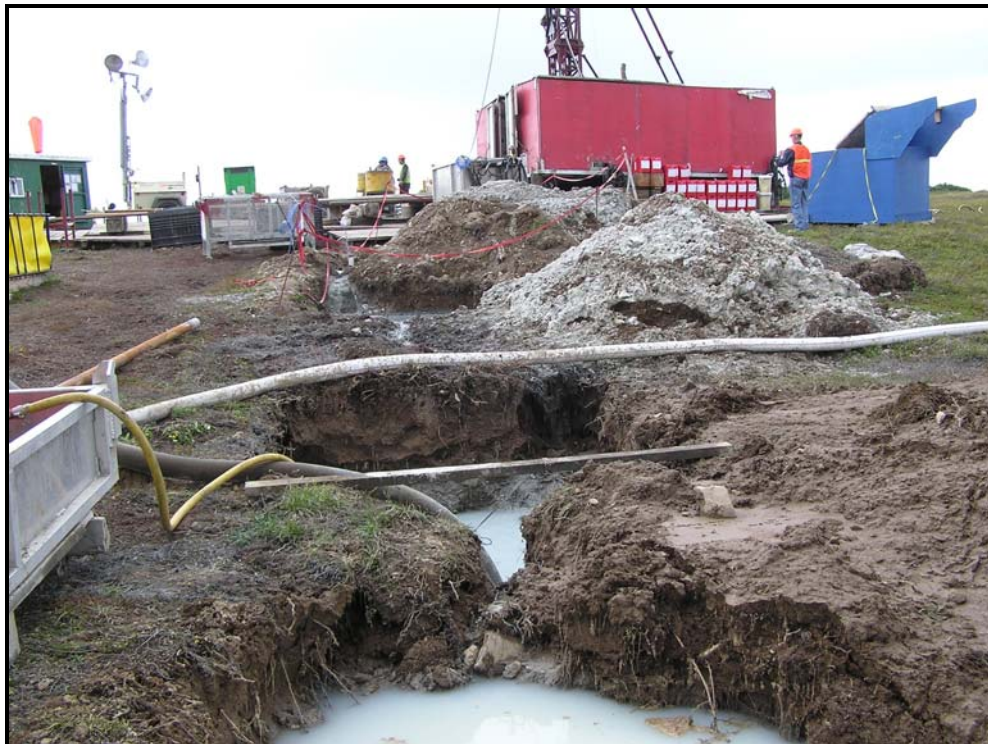
Figure 26: Sumps for Drill Rig # 4.
