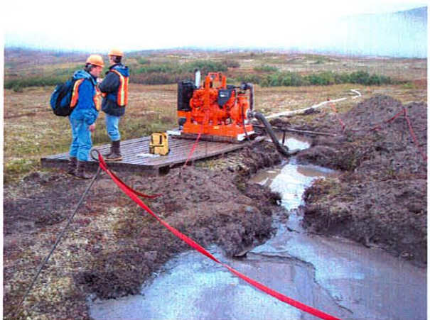
Figure 4. Series of three sump pits with Godwin pump and discharge to uplands.
