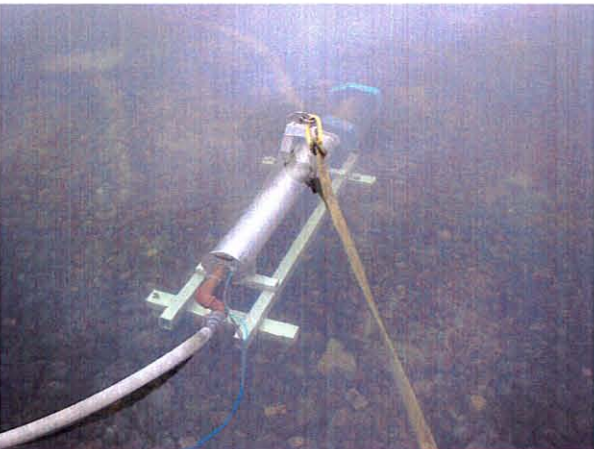
Figure 5. Water intake pump and screen.
