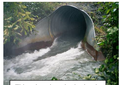
This culvert is undersized and the water velocity is too fast.
