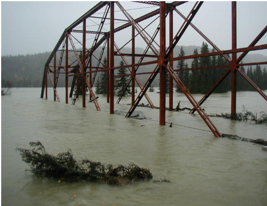
FIGURE 4-31. Flood in Iliamna River on October 1, 2003 (GS 3a).
